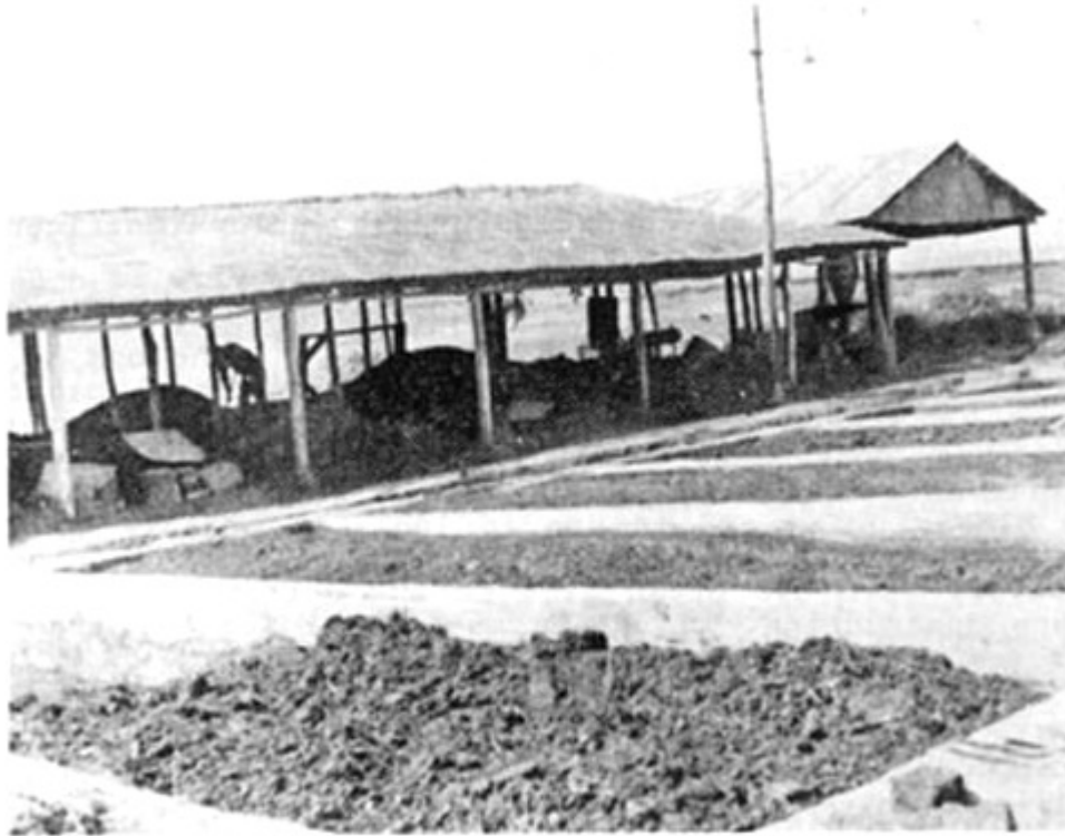
Plate 20 Pits constructed above ground for refuse-night soil composting. Hammer mill for crushing and sieving facilities under cover at rear Source: Gotaas (1956) and van Vuren (1949)
